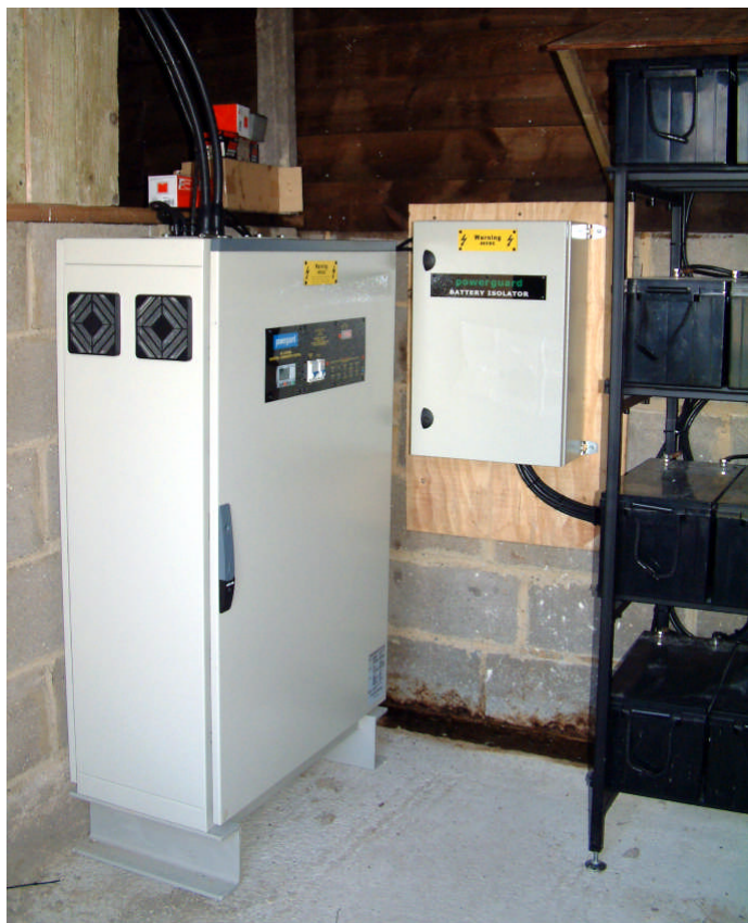
A TYPICAL INSTALLATION SHOWING THE PS SYSTEM, BATTERY ISOLATOR AND PART OF THE BATTERY BANK.
